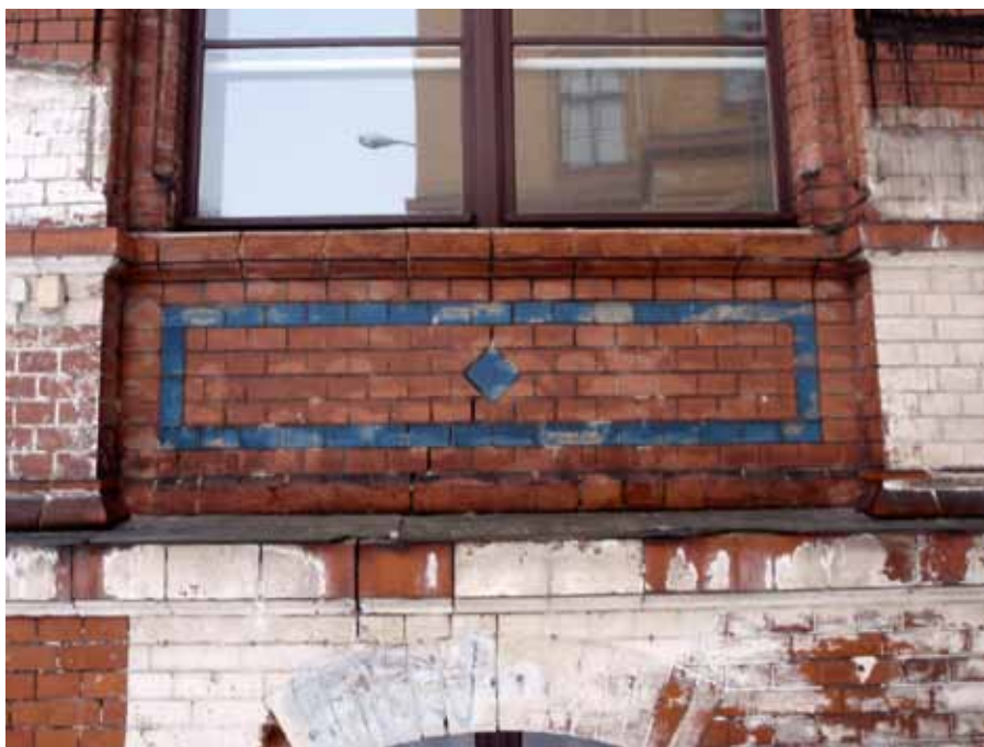
Fig. 10. White paint and crack below the window of the NIII façade; photo by author.
