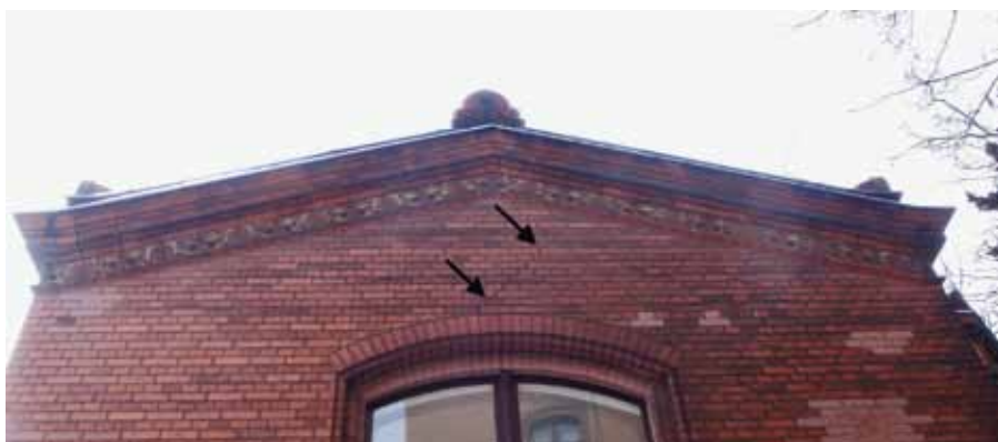
Fig. 11. Structural damage above the window of the NIII façade possibly caused by the addition of a garage; photo by author.
